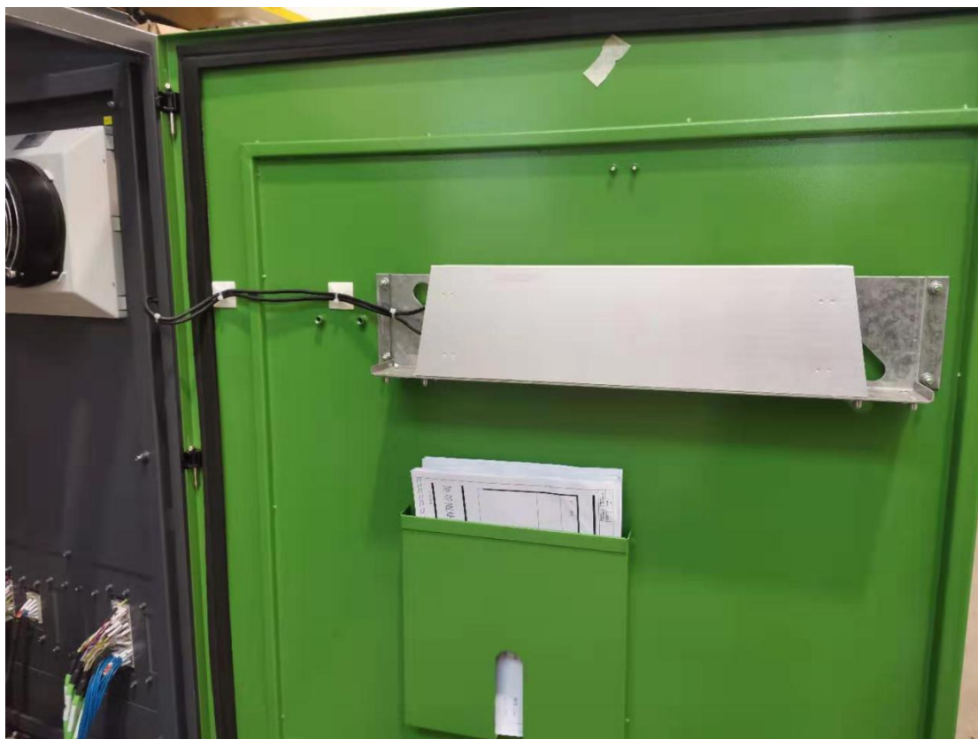
Detailed wiring and layout in cabinet 6
