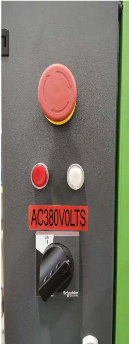
Electric cabinet switch and panel button
