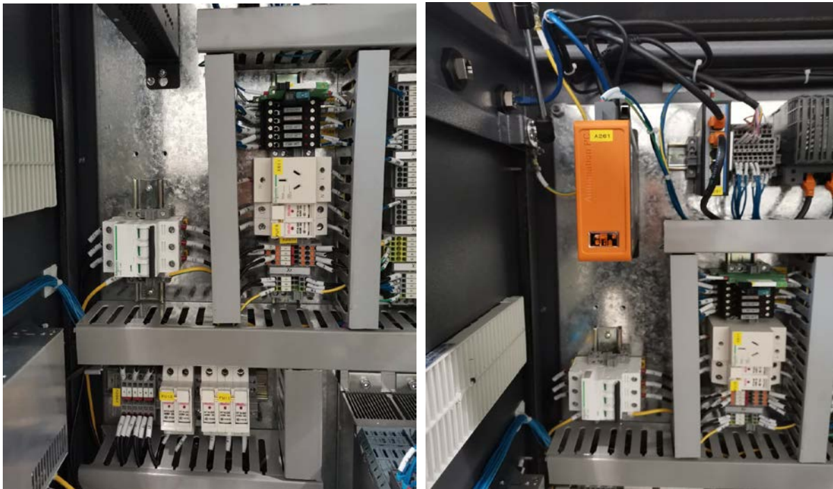
Detailed wiring and layout in cabinet 2
