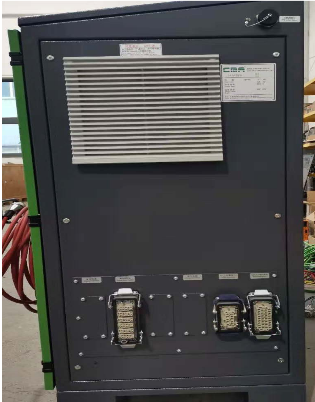
Installation and layout of relevant components on the right side of electric cabinet
