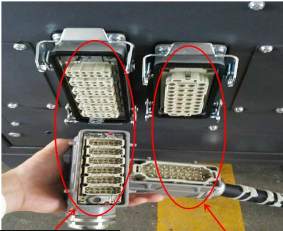
Plug-in socket of electric control cabinet encoder line
